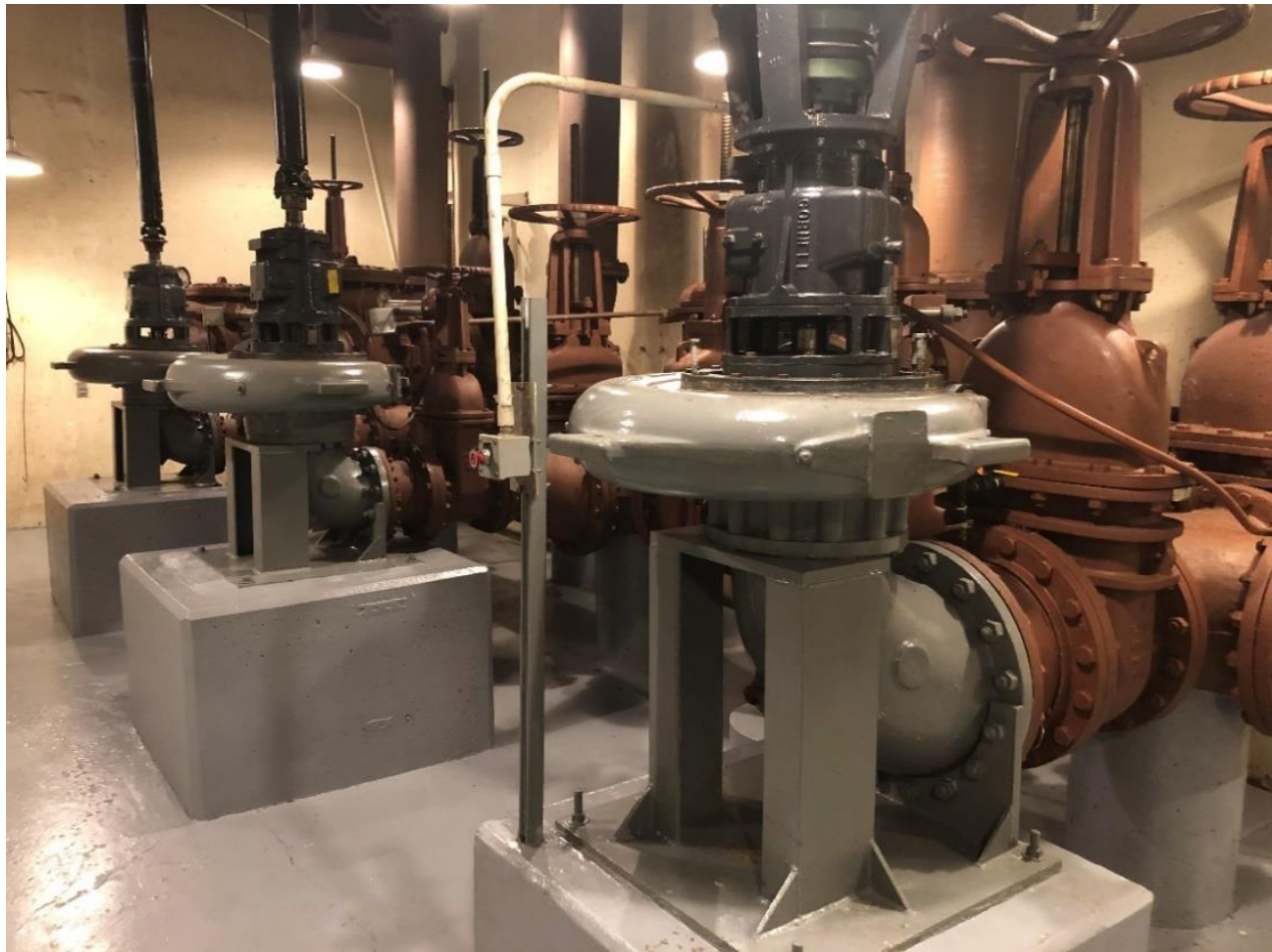
Photo 1 – Pumps at the Katrina Road Pump Station
